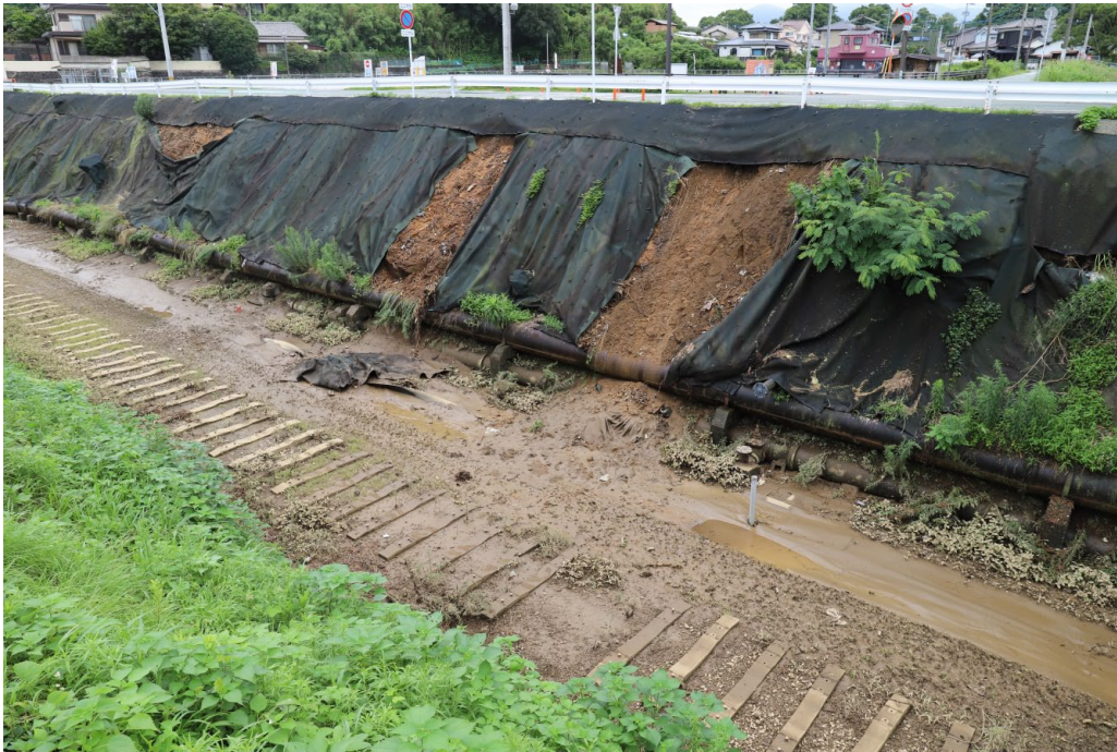
Miike Coal Railway: Photo of damage status
