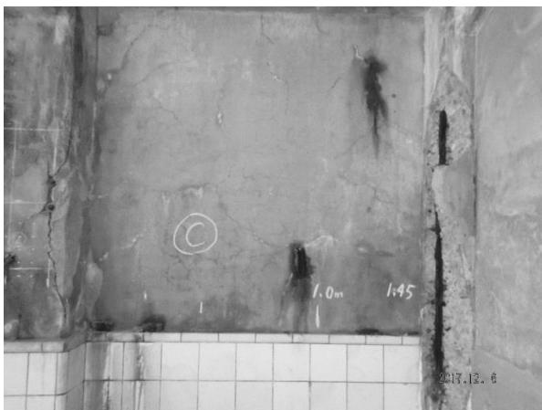
Photo 2-4-98. explosion and corrosion; on base lines A and 2 intersection, Level 1
