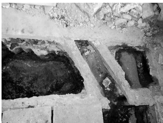
Photo 2-4-89. Exploratory Drilling Site ②, examination of iron pipe and Layer 2, viewed from south
