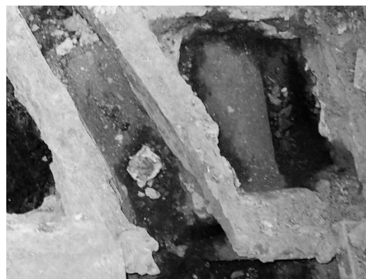
Photo 2-4-90. Close-up (iron pipe)
