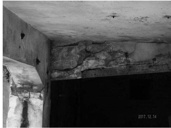
Photo 2-4-101. Cracks and falling-off; Beam 2G3A, Level 2
