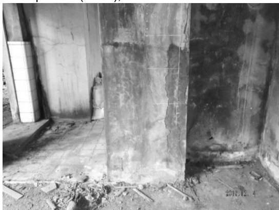
Photo 2-4-97. Cracks; column on base lines C and 2 intersection, Level 1
