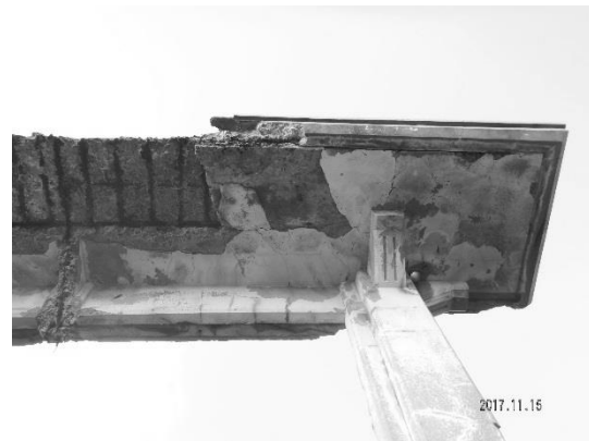
Photo 2-4-103. explosion; back side of eaves
