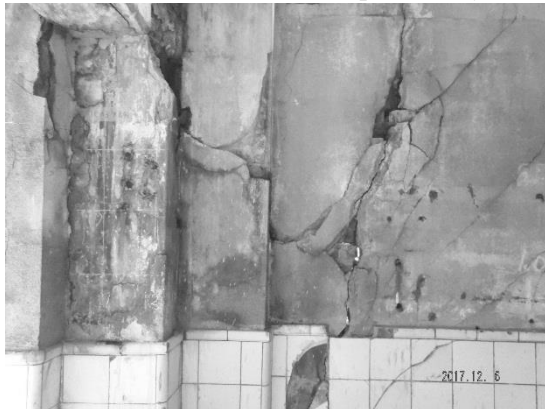
Photo 2-4-95. Mortar cracks and falling-off; plane C (South), inner wall
