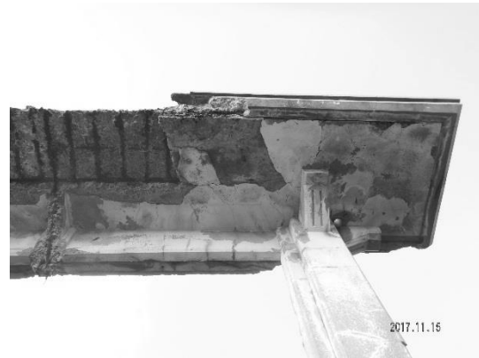
Photo 2-4-103. explosion; back side of eaves
