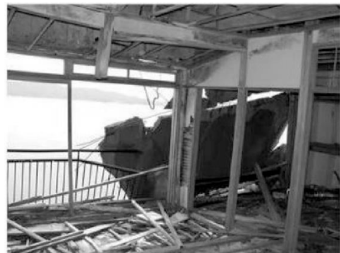
Photo 2-4-124 Interior fixture deterioration condition
