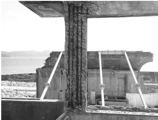
Photo 2-4-102. explosion; Eaves on base lines C and 2 intersection
