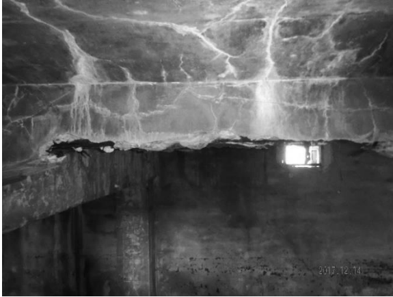
Photo 2-4-100. explosion and corrosion; Beam 2G1Aa, Level 2
