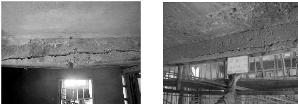
Photo 2-4-120 Deterioration level III
