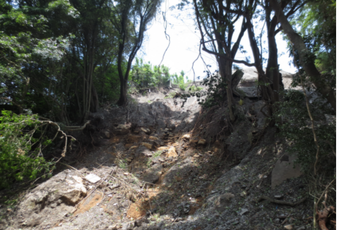
(4) Midslope of landslide (photographed July 9, 2019)
