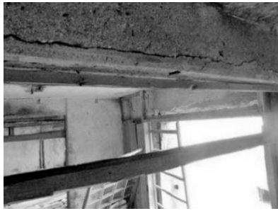
Damage degree III
