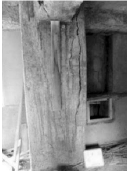
Column: Damage degree III
