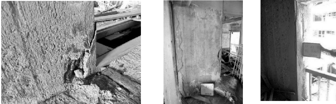
Photo 2-4-119 Deterioration level II
