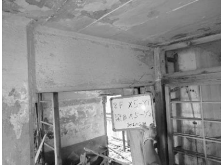
Photo 2-4-118 Deterioration level I
