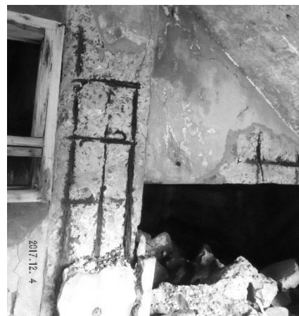
Photo 2-4-99. explosion and corrosion; on base lines B and 1 intersection, Level 1
