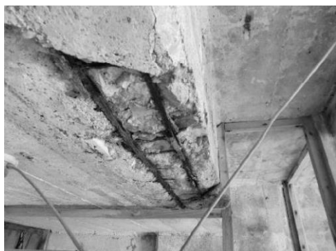
Photo 2-4-121 Deterioration level IV
