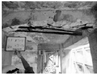
Damage degree IV
