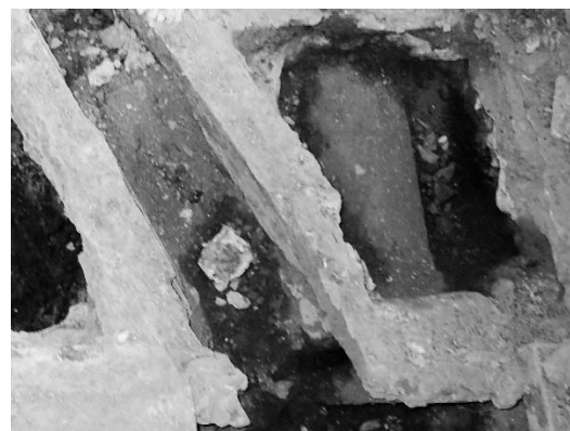
Photo 2-4-90. Close-up (iron pipe)
