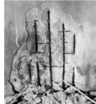
Wall: Damage degree IV
